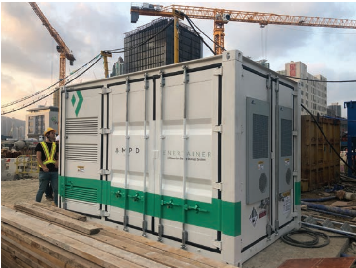
The energy container, or 'Ener-tainer', uses a very small amount of electricity to charge but can easily power a tower crane due to the high peak demands but long idle times
